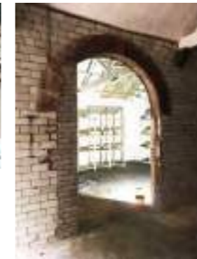
Print workshop External - stone (NW & SW) & brick (SE) Internal - glazed brick (NW shed), painted brick (SE shed) Heritage significance - Medium social/cultural significance Dinwiddie print studio
