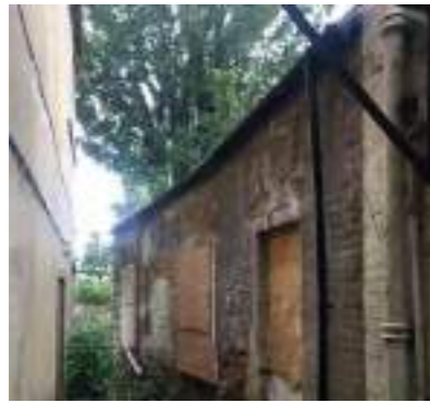
South west end (single storey) External - stone, largely altered with brick. Internal - mostly brick. Heritage significance - Low
