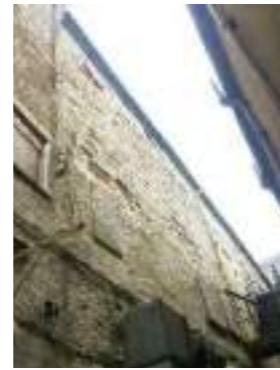
Main section (all storeys) External - stone (spalled face and painted) Heritage significance - Low
