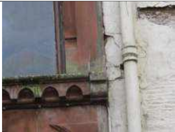
5.15 abutment cracks to 113
