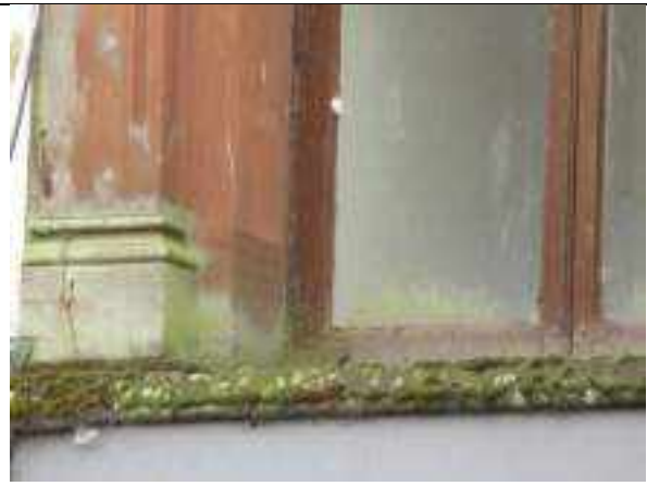
5.16 cracked pilaster above shop front
