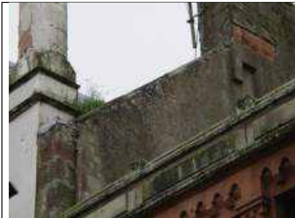
5.13 parapet and cracked stone buttress at gable
