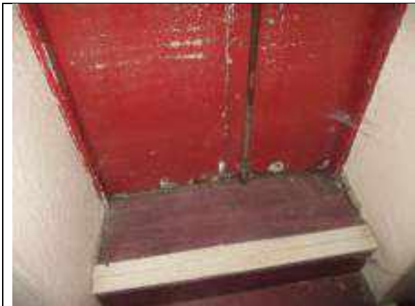
5.19 rot at lower edge of dor
