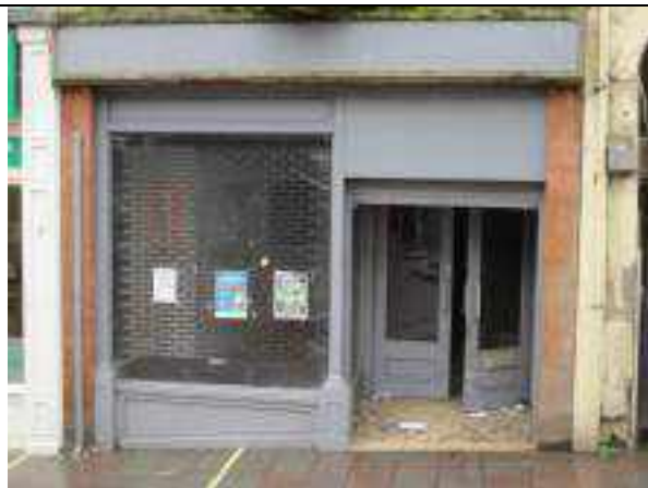
5.17 timber shop front
